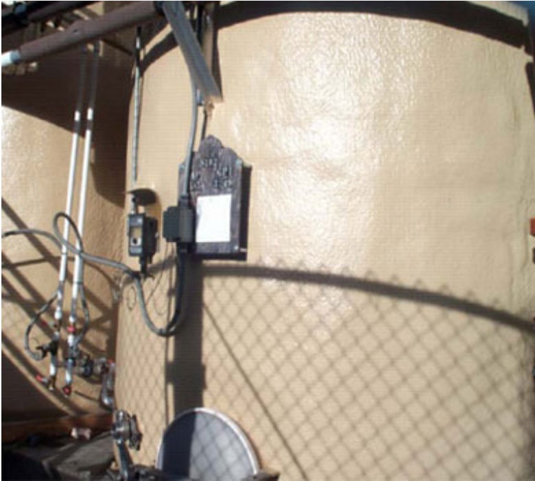
Phoenix Coatings ability to adapt the application to any tank style is an art form accomplished by true craftsmen.
